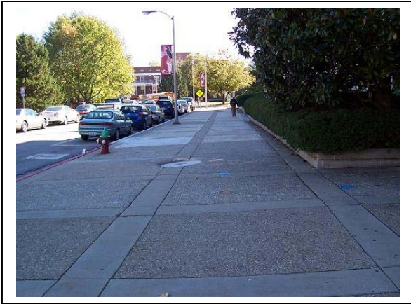
The sidewalk on University Drive masks several safety hazards.
