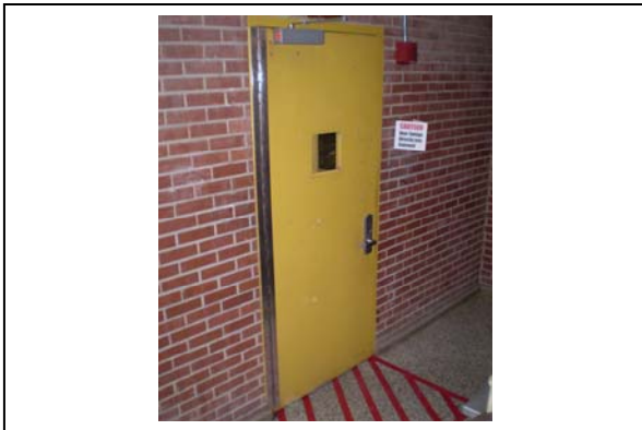
Close-Up of Door Hazard Warning System: Shown installed in the dangerous stairwell with red warning tape at door swing and three dimensional caution sign.
