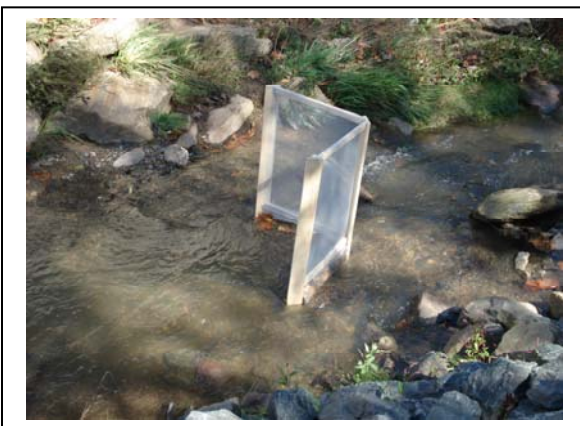
System catching sediment and debris near major water run-off.
